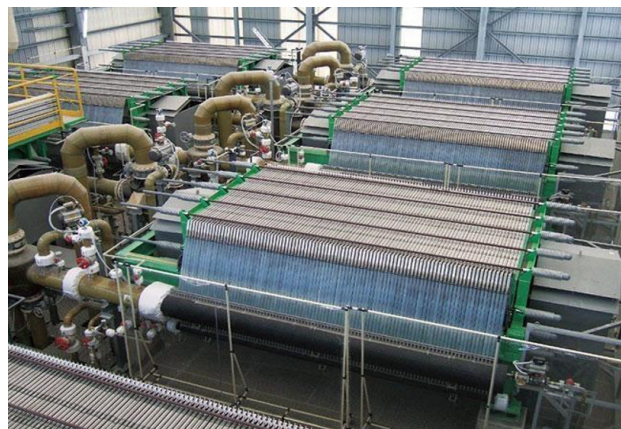
Fig. 5.13: Typical large scale electrolyser set-up (Thyssen-Krupp 7 )
