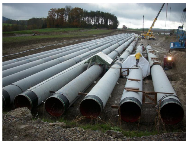
Fig. 5.9: Natural gas tubular storage Urdorf (Jauslin Stebler AG 4 )
